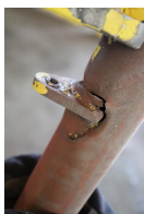
(Rudder damage caused by wind)
